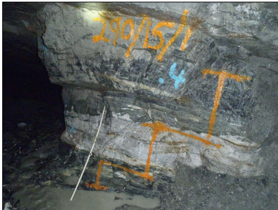
Figure 8-14 Marked-up sample location on the 300 SB East Level at the top of stope 290-15 (western side) with metre rule for scale (source: SRK ES 2016)
