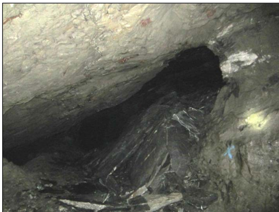
Figure 23-3 Significant hanging wall failure from stope 510-27 where rock slabs have fallen into the drive (source: SRK ES, 2016)
